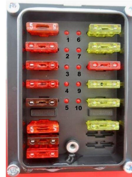
Picture 87: fuse box.
